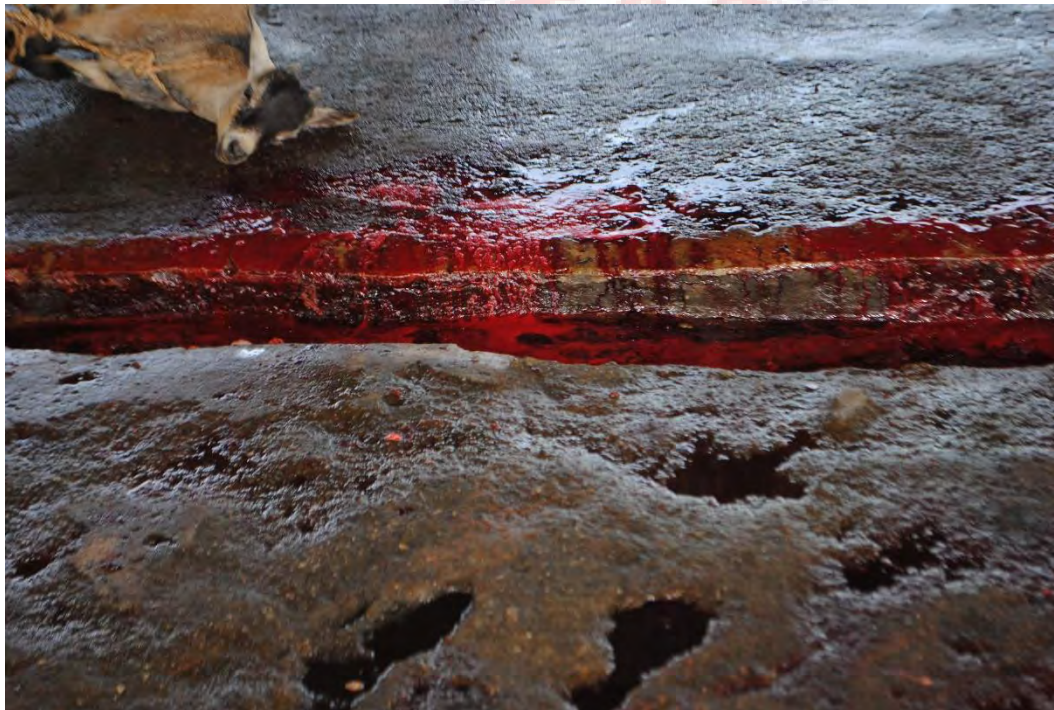
Rough surfaces of the working floor
