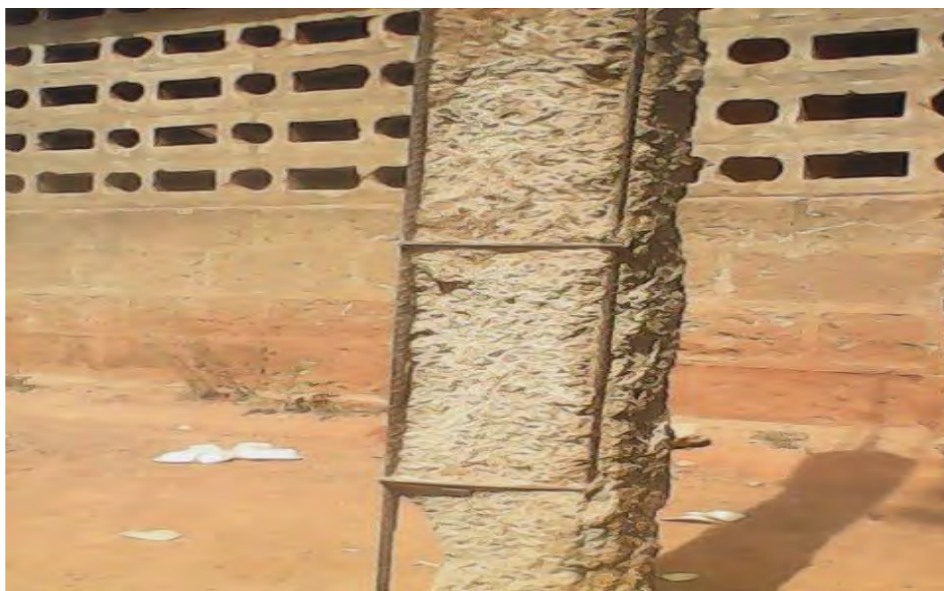
Figure 4.9 defected pillar at Charia M/A Block ‘B’ junior High School
