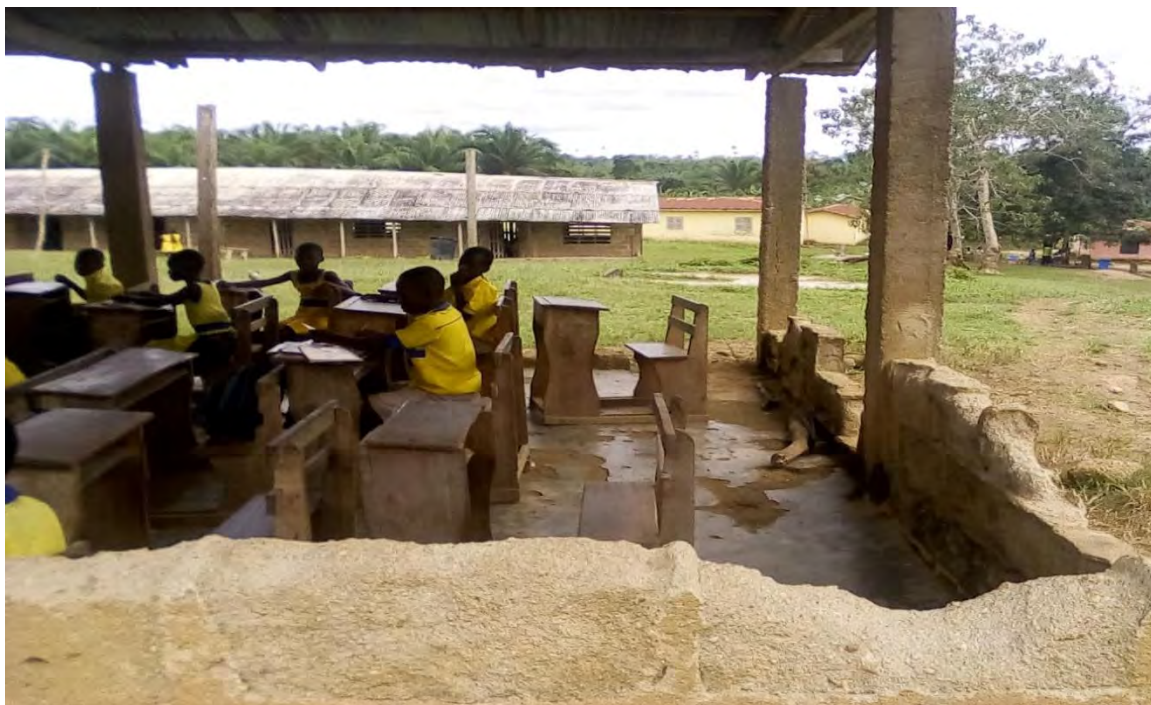
Figure 4.25 Collapsed walls of Akim Wenchi Methodist Basic School
