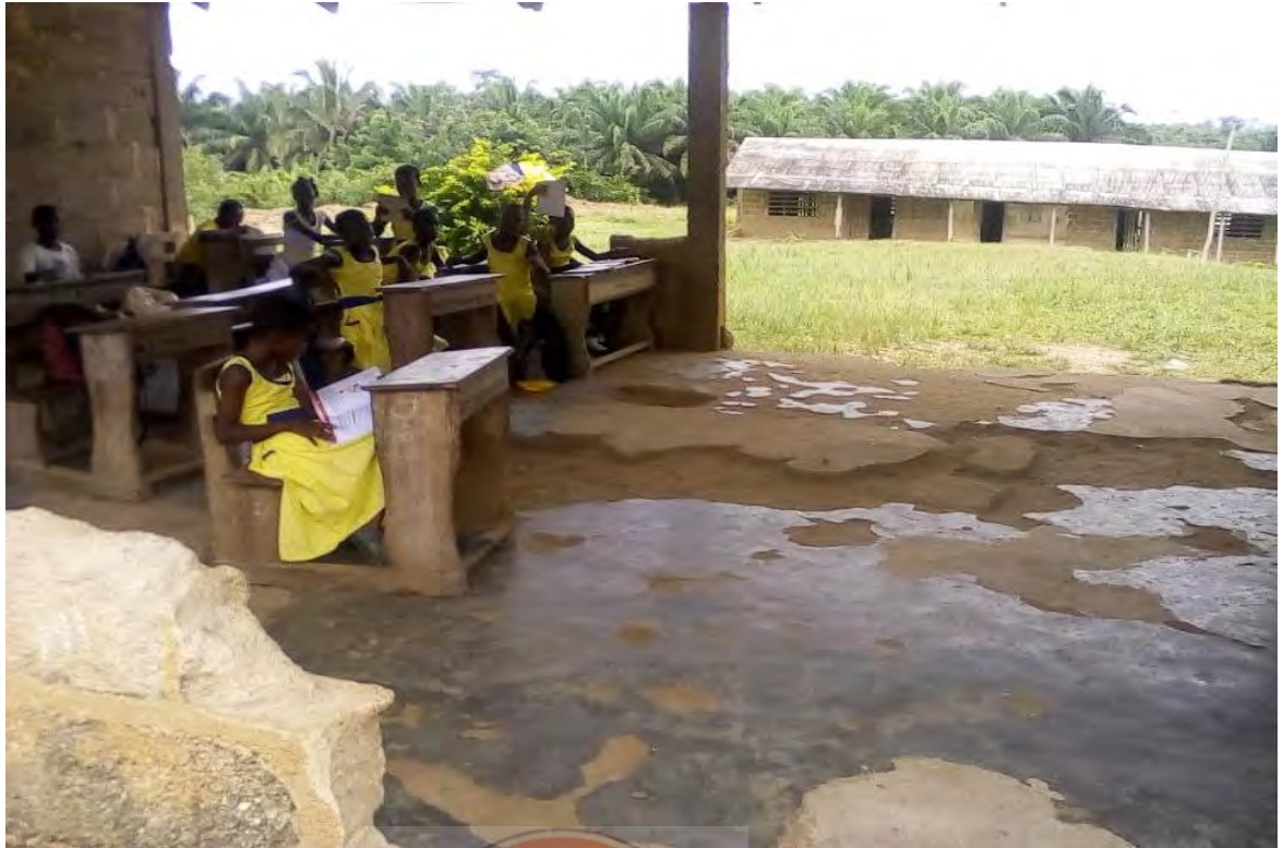
Figure 4.26 Peeled off floor of Akim Wenchi Methodist Basic School
