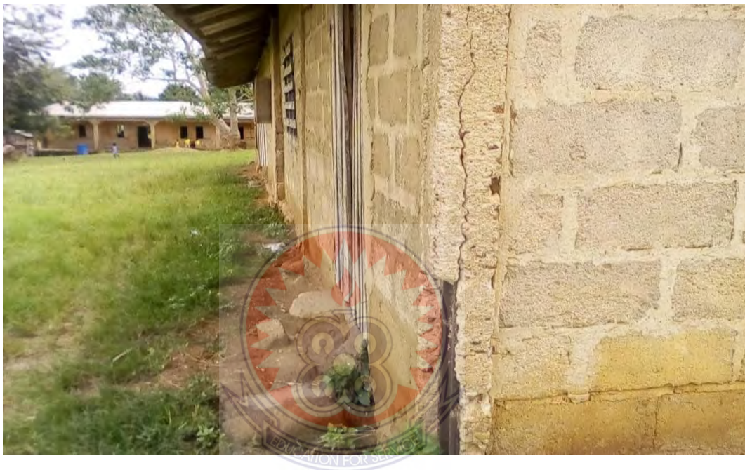
Figure 4.18 Cracked corner column of Kusi Methodist Basic School exposing the reinforcement.
