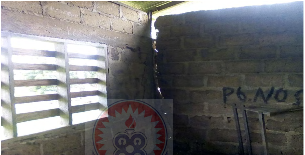
Figure 4.23 Deep crack on wall at Addaekrom D/A Basic School which has separated the two adjacent walls.
