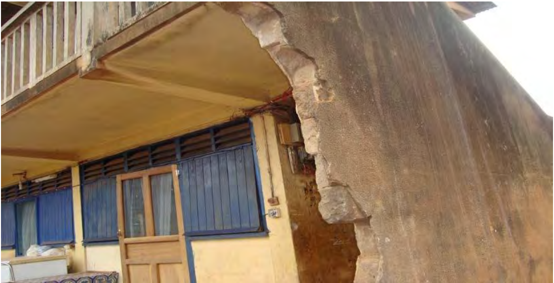
Fig 1 Broken Walls at Sagnarigu District Tamale.
