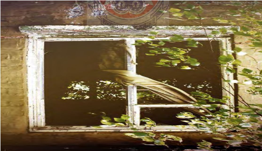
Fig 2 Broken windows at Sagnarigu Tamale.
