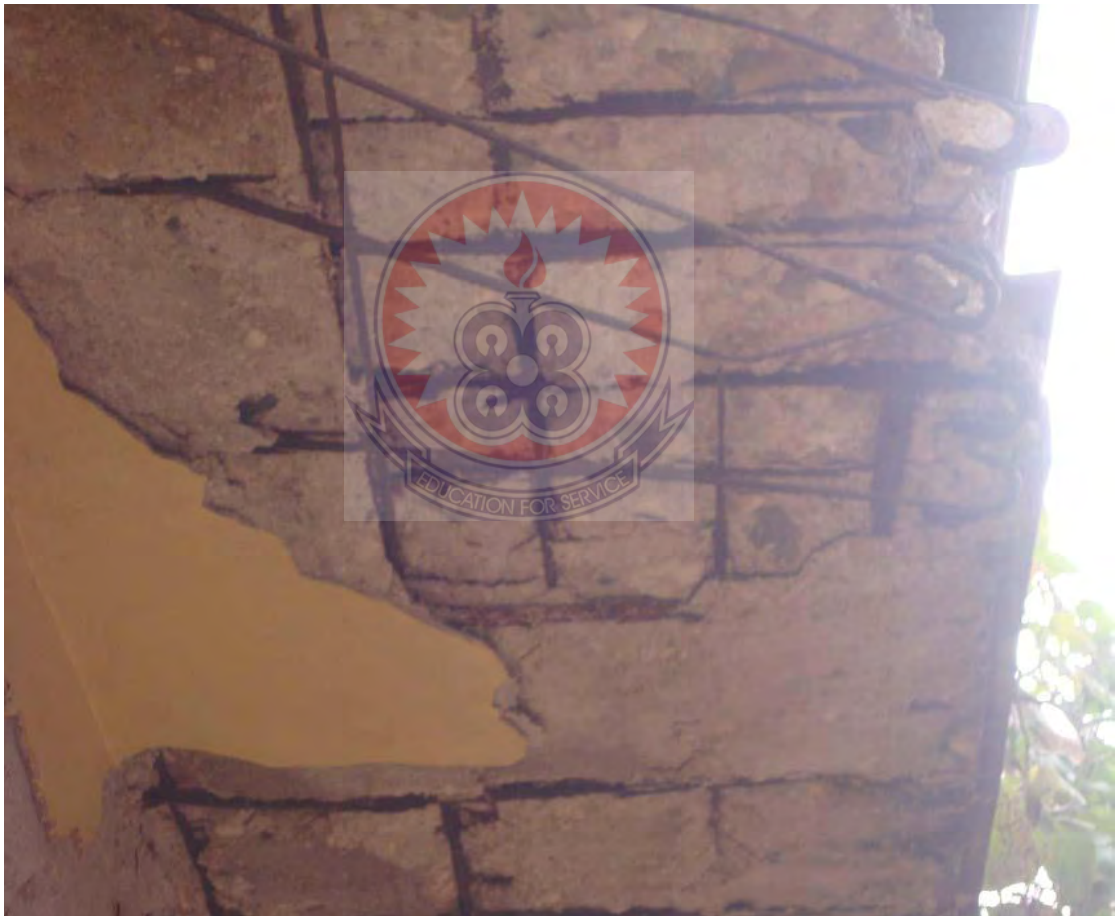
Figure 4. 1 Peeled – offs/cracks of roof at G. E. S Tamale.
