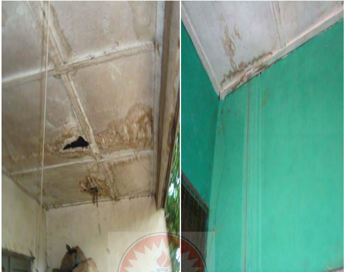
Figure 4.2 leakages of roof at BDJHS Tamale.
