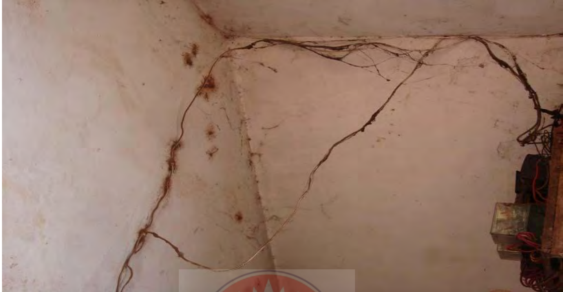
Figure4. 4 Electrical wires hanging on buildings at Tamale.
