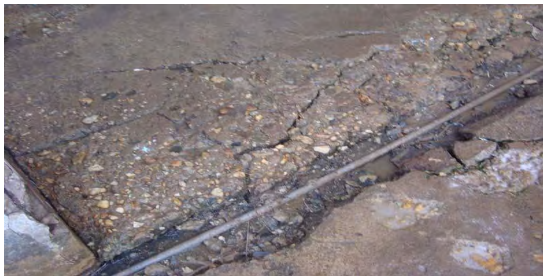
Figure 4.3 Floor cracks at G. E. S. Tamale.
