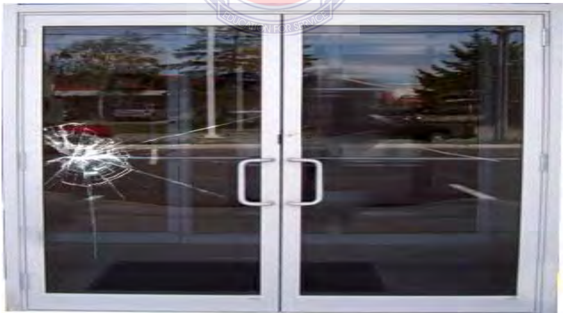
Figure 4.2 Broken door at G. E. S Tamale.
