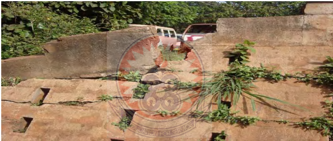
Figure 4.2 Broken down walls of buildings of policymakers at Tamale.
