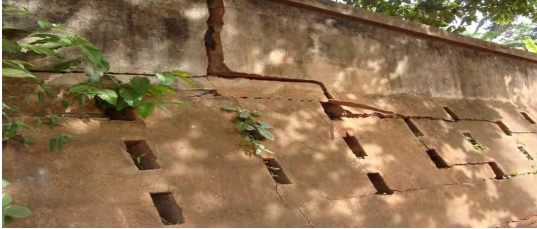
Figure 4.1 Broken down walls at G. E. S Tamale.
