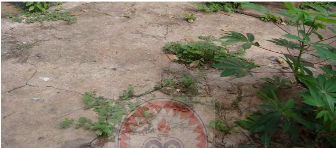
Figure 4.2 Floor cracks at G. E. S. Tamale.
