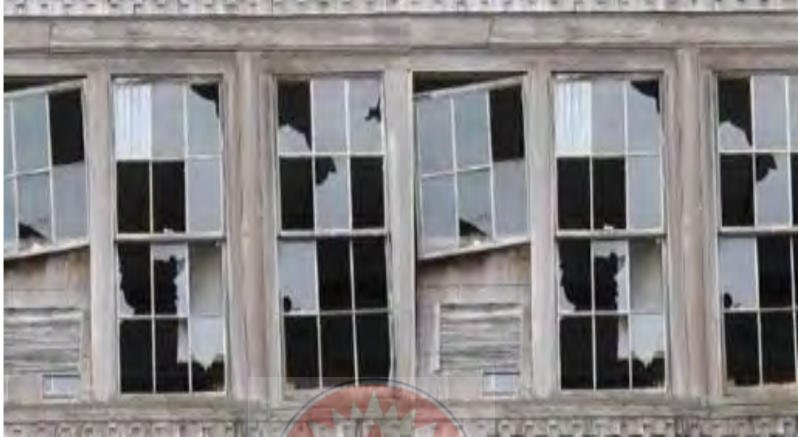
Figure 4.1 Broken window of buildings of Policymakers at Tamale.
