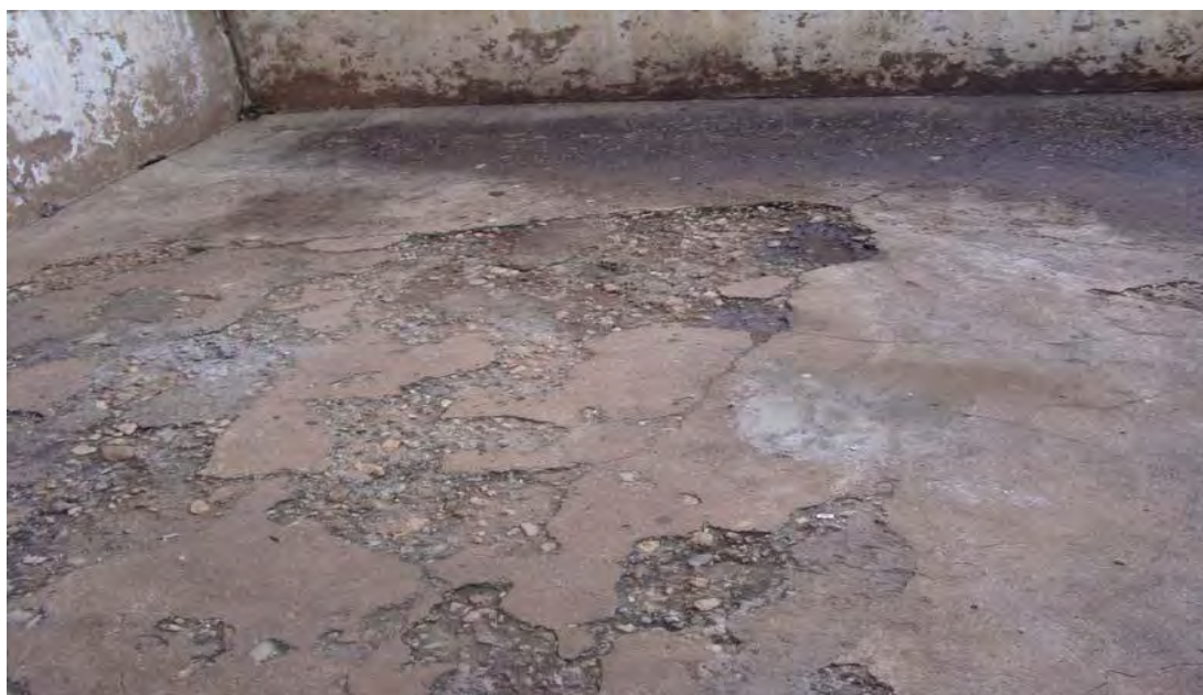
Figure 4. 1 Floor cracks at BDJHS Tamale.
