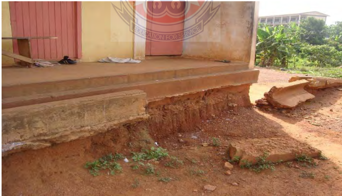
Figure 4.3 foundation exposed / hanging at G. E. S Tamale.
