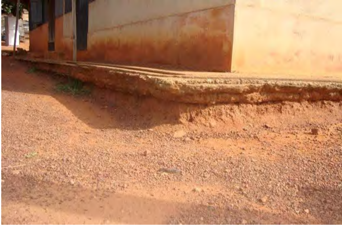
Figure 4. 2 Foundation exposed at BDJHS Tamale.
