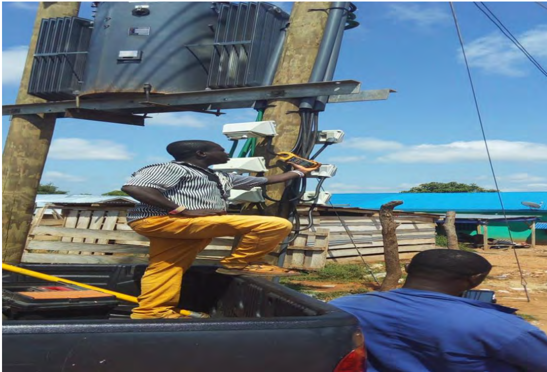
Figure 1.1: A NEDCo Staff Monitoring a Transformer Load Current Manually (Source: TechimanNEDCo Diary)
