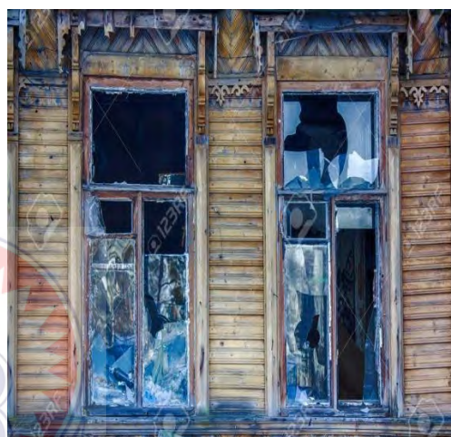
Figure 4. 5: Glass window breakages Source: Field Work, 2018
