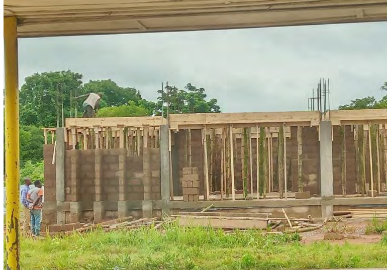
Figure 4.3: Observation at Bamahu, it was revealed that workers does no wear helmet, overall, safety boot and hand gloves which exposed them to danger.
