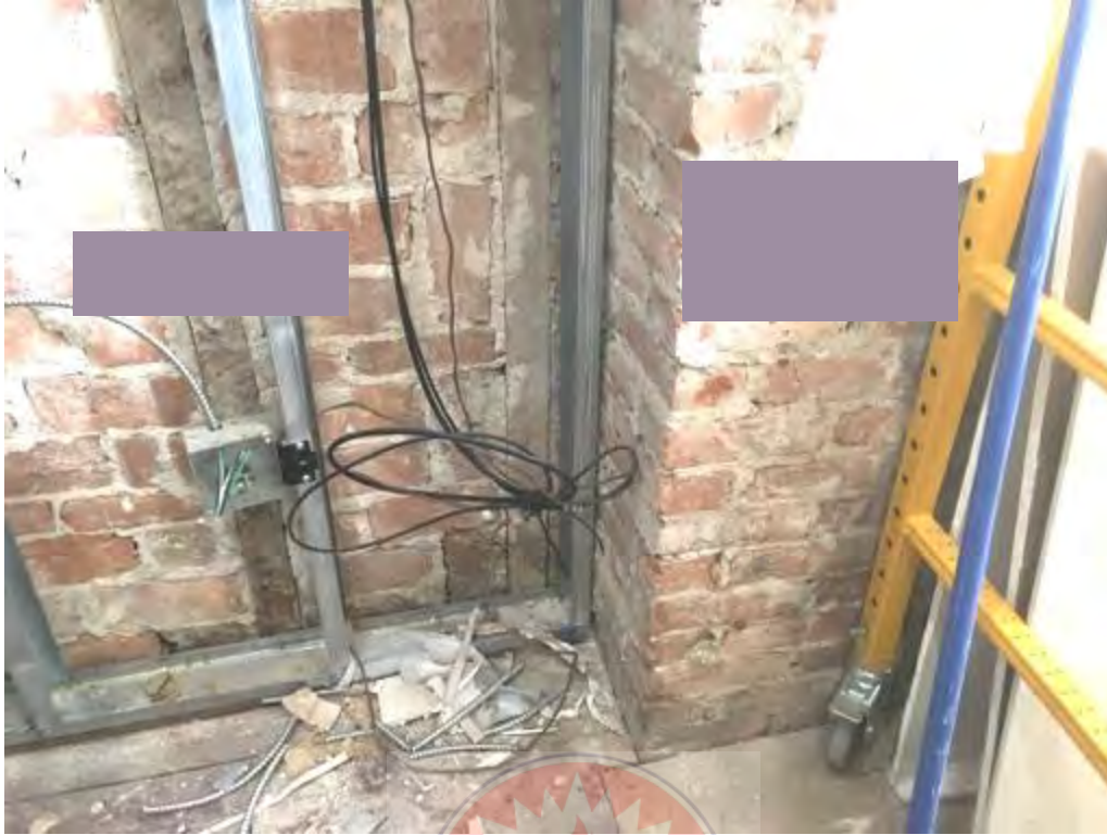
Figure 4.3 Exposed Electrical Cables and Fittings at the Basic Schools at Sogakope.
