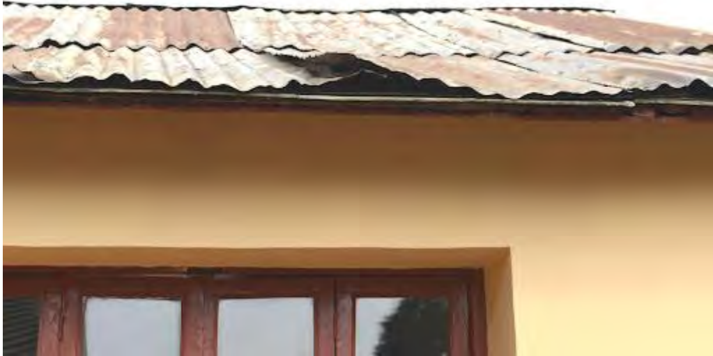
Figure 4.1 Leaking and Rusting of Roofed Members at Basic School at Sogakope.
