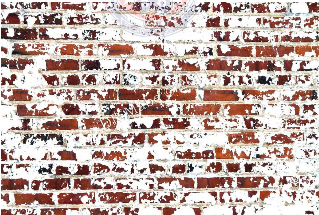
Figure 4.4 Dilapidated Structures at the Audit and National Service Office at Sogakope.
