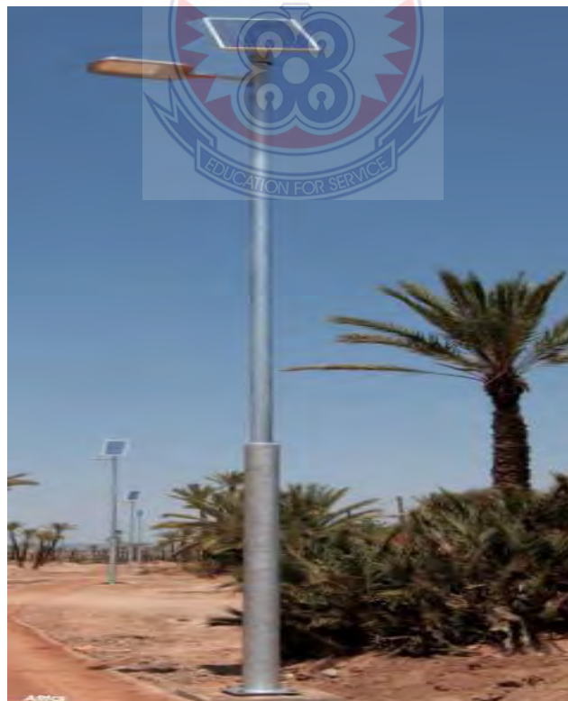
Figure 2.8 Solar powered street light
