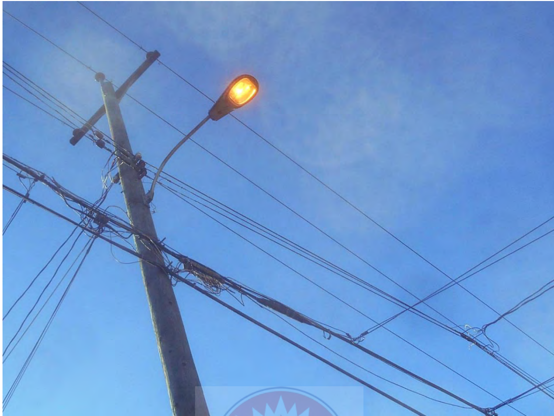
Figure 2.6 Traditional Street light
