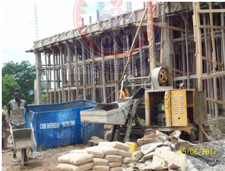
Fig 4.8 Cement Bags Left On Damped Ground without Pallets at On-Going Hall Of Residence At UDS Wa
