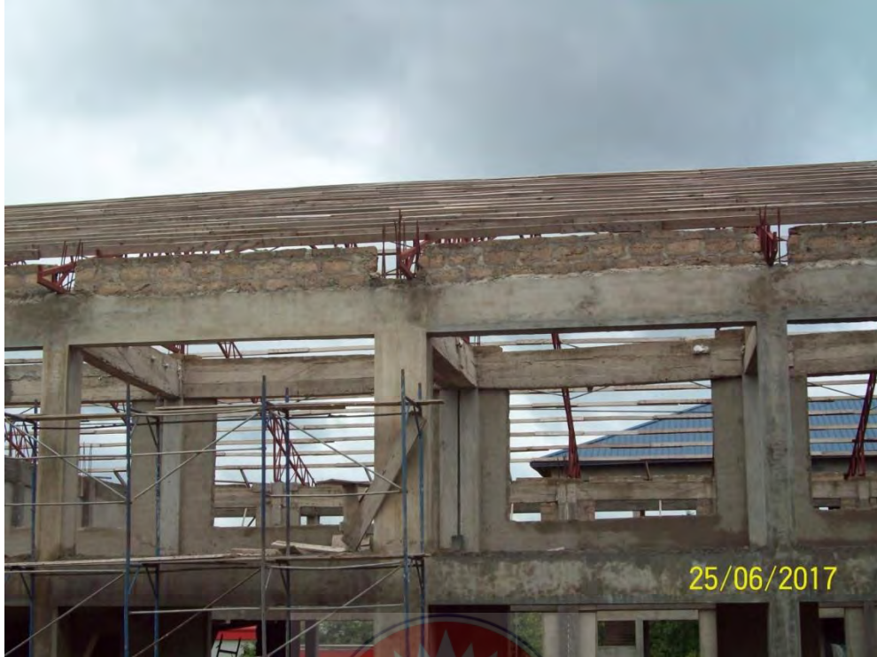
Fig 4.12 Timber purlins exposed to the vagaries of the weather of on-going lecture hall complex
