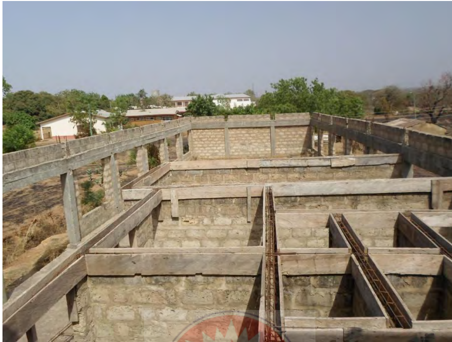
Fig 4.1 Reinforcement bars in lintel formwork at N.J Ahmadiyya College of Education on-going Multi-Purpose Auditorium Complex
