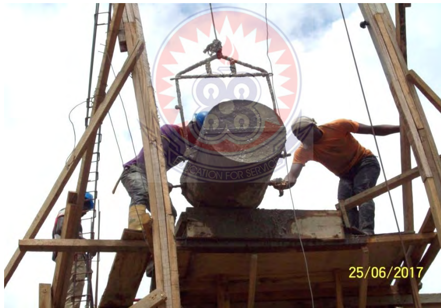
Fig 4.10 A concrete hoist mechanical used to pour concrete mixture on a slab
