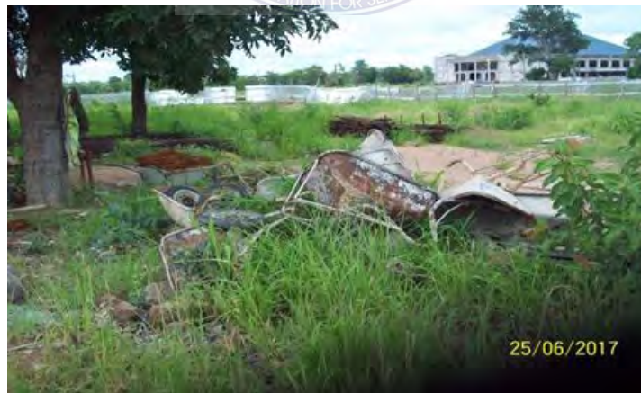
Fig 4.6 wheelbarrows and reinforcement iron rods at the vagaries of the weather at library block complex at UDS Wa Campus
