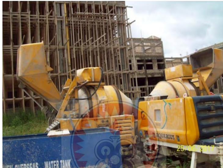
Fig 4.5 concrete mixer machine being exposed to weather without
