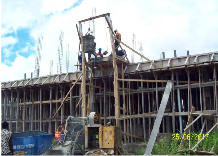
Fig 4.7 Construction in process without regards to operatives safety at UDS Wa Hall of Residence construction site
