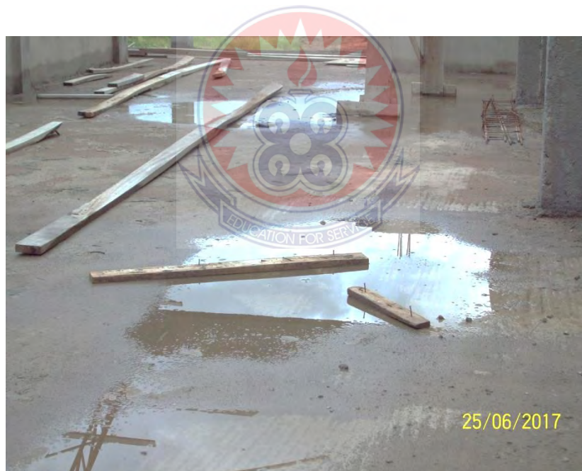
Fig 4.11 water stacked on a decked slab due to uneven surface at the on-going construction of 3-storey lecture hall complex at UDS-Wa
