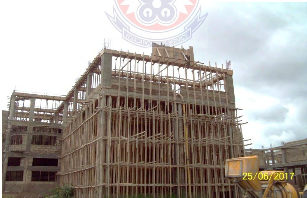
Fig 4.4: Wooden props used to support slabs at U.D.S Wa campus on-going library block complex
