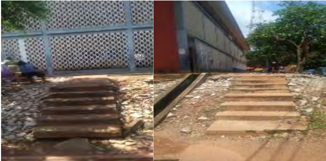
Fig 4.18: These entrants at the Adum Ministries is dilapidated and dangerous to the users including the disabled persons (Source: field survey 2018)
