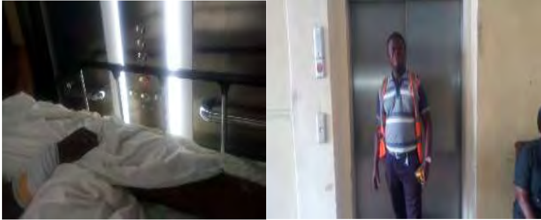
Fig 4.8 Majority of the elevators in A, B, C and D blocks are nonfunctional. A source of worry for the physically challenged. (Source: field survey 2018)
