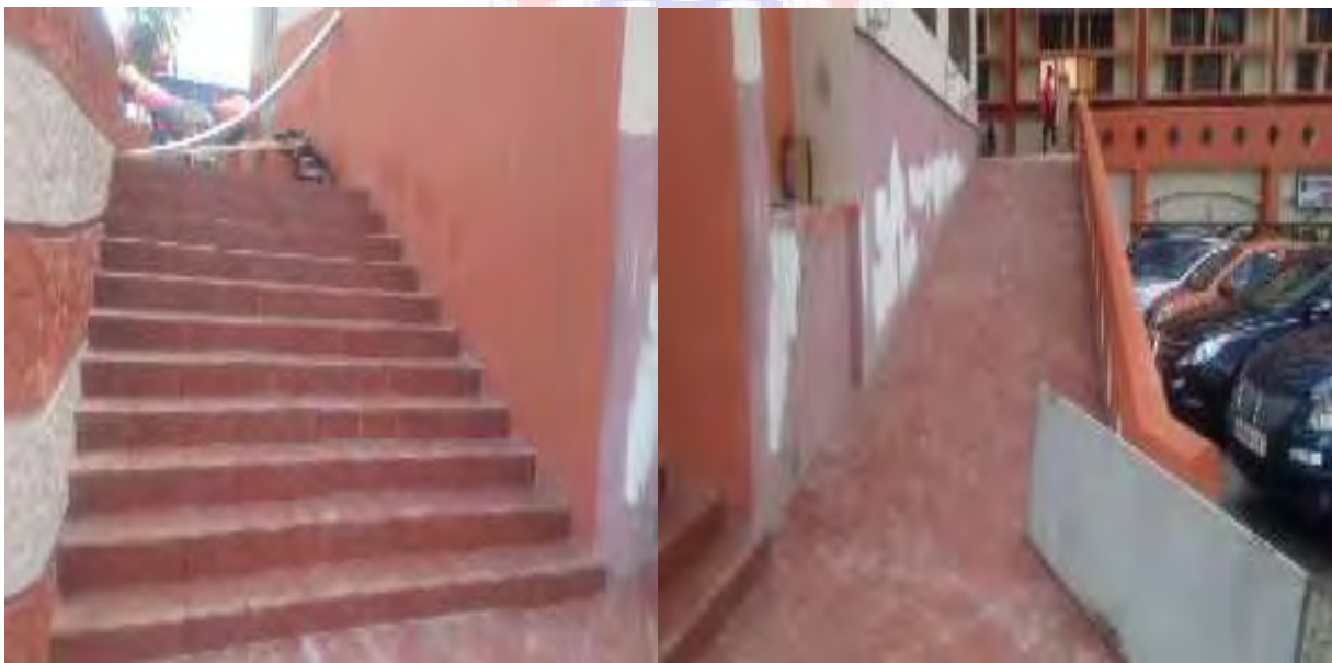
Fig 4.16: The ramp at Main entrance at the Electricity Company at Adum, Kumasi is too smooth and steep for the disable (Source: field survey 2018)
