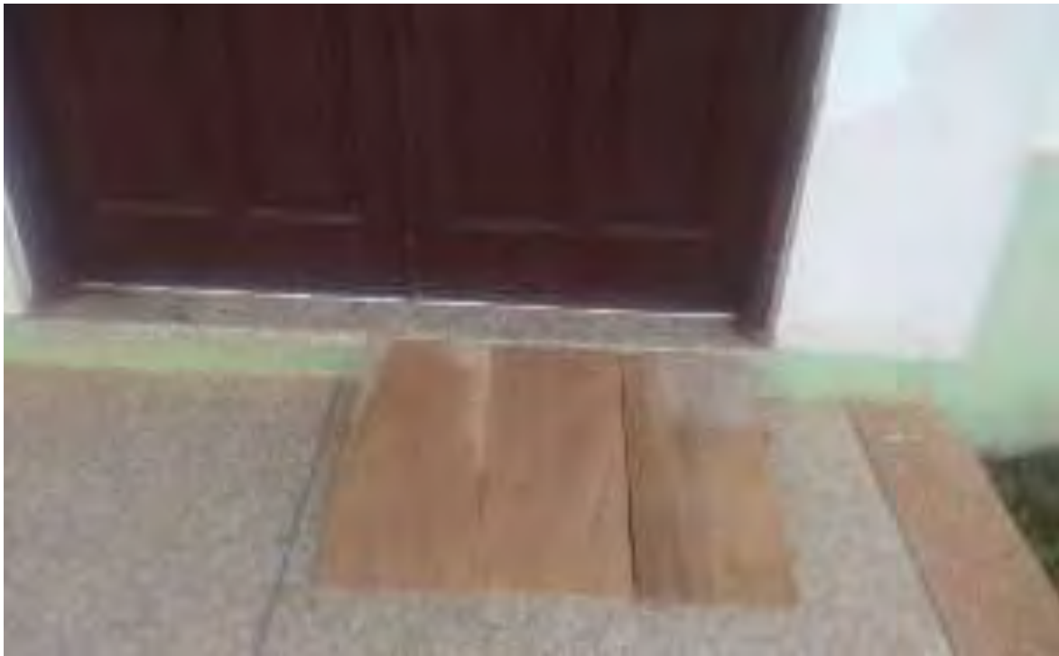
Fig 4.20: This temporary placed at the access route to the new auditorium to make accessible to the disable is inadequate. (Source: field survey 2018)
