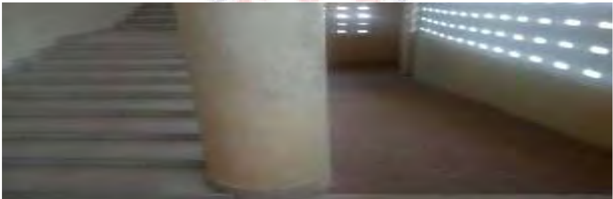
Fig4.13: The Male ward in Sunteso hospital has ramp along the steps and ramp housed in the stairwell up to the first floor. (Source: field survey 2018)
