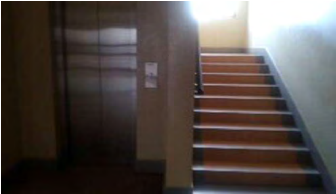
Fig 4.18a: The elevator at the legal aid building, Kumasi is faulty.
