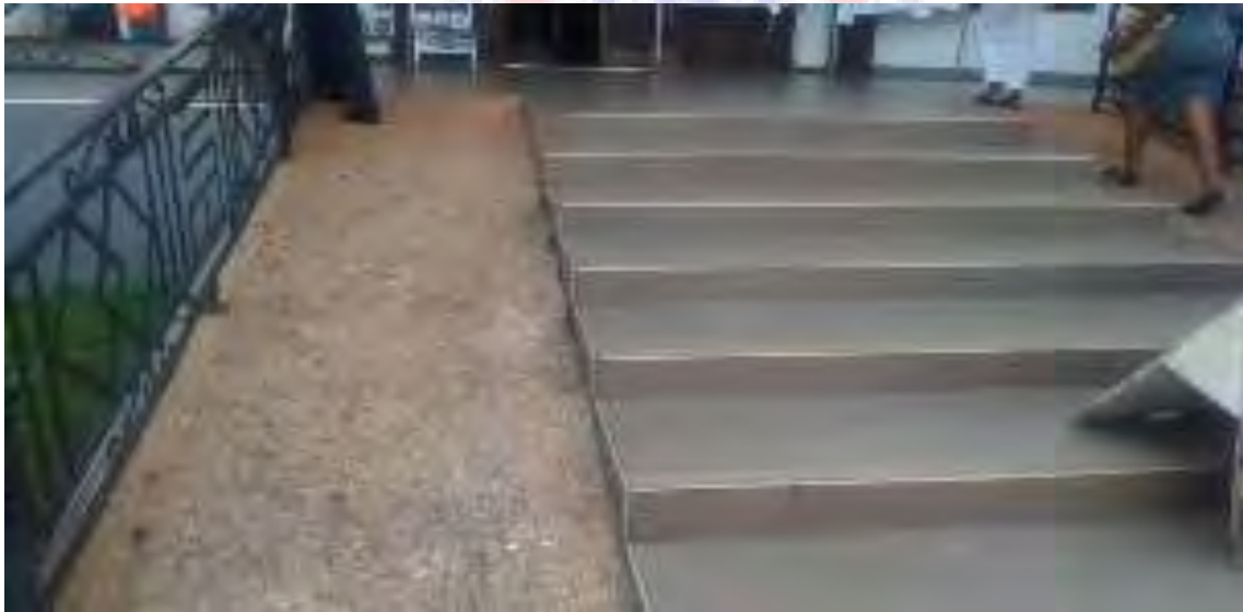
Fig 4.18b: This ramp at the entrance of the legal aid building, Kumasi is too narrow in width and steeply for comfortable of the disabled (Source: field survey 2018)
