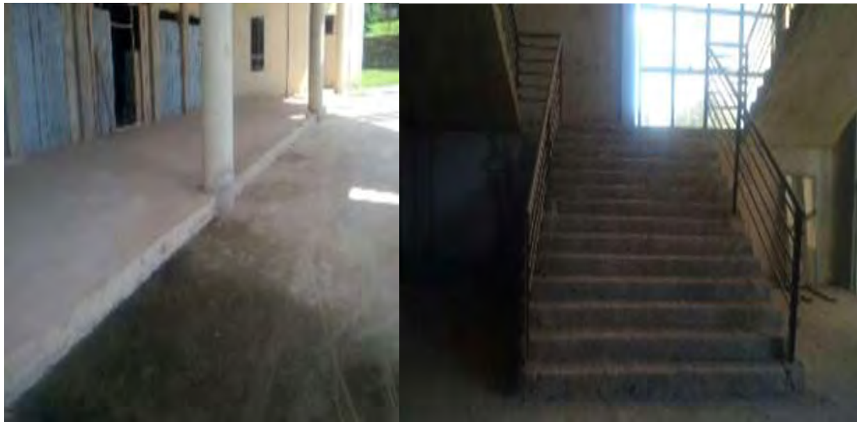
Fig 4.25: The main entrance and interior of the auditorium building under construction at UEW-Kumasi lack provision for the disabled (Source: field survey 2017)
