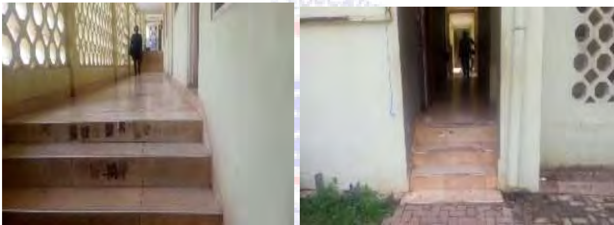
Fig 4.23: Corridors to the Opoku Ware Hall lacks provision to the disabled. (Source: field survey 2018)
