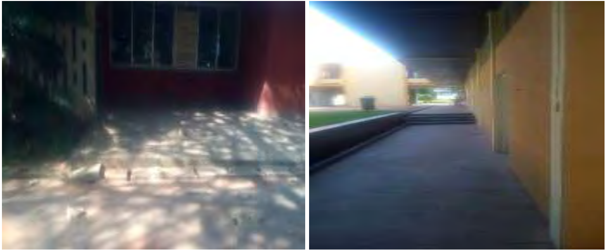
Fig 4.27: The faculty of Architecture building at KNUST, Kumasi lacks provision for the disable at both entrance and corridors (Source: field survey 2018)
