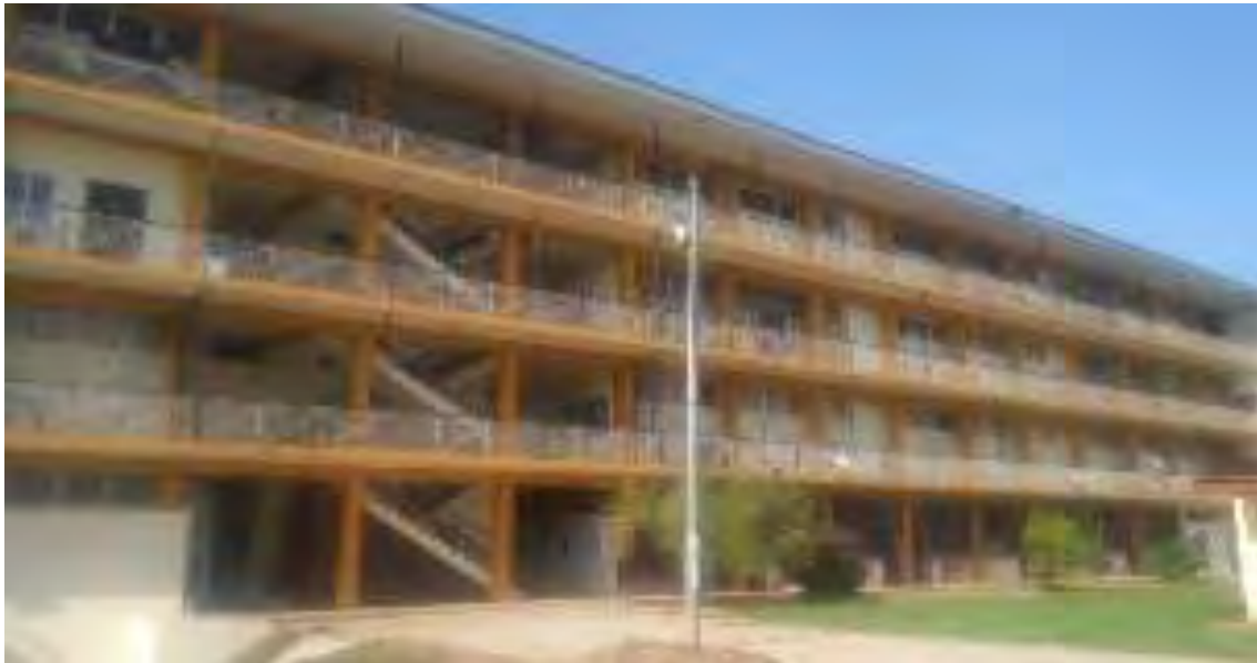
Fig 4.26: Faculty of Social Sciences building at KNUST, Kumasi. Lacks provisions for both horizontal and vertical movement for the disabled (Source: field survey 2018)
