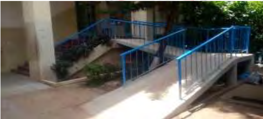
Fig 4.9 The gradient for this ramp constructed recently ear nose and throat center of KATHHT is too steeply (Source: field survey 2018)
