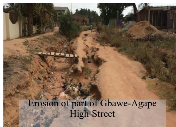
Figure 20: Flooding in Ablekuma and the eroded part of Gbawe-Agape High Street
