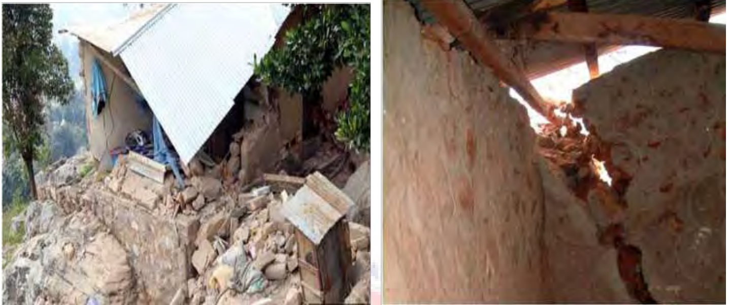
Plate 4.3: Aftermath of March, 2019 earth tremor at the hill top and last stop area
