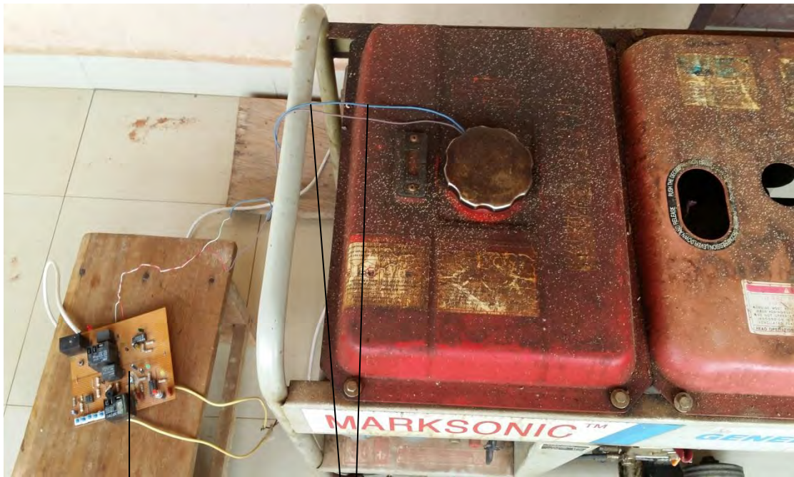
A Picture showing the Timer Switch Connecting wires into the fuel tank.
