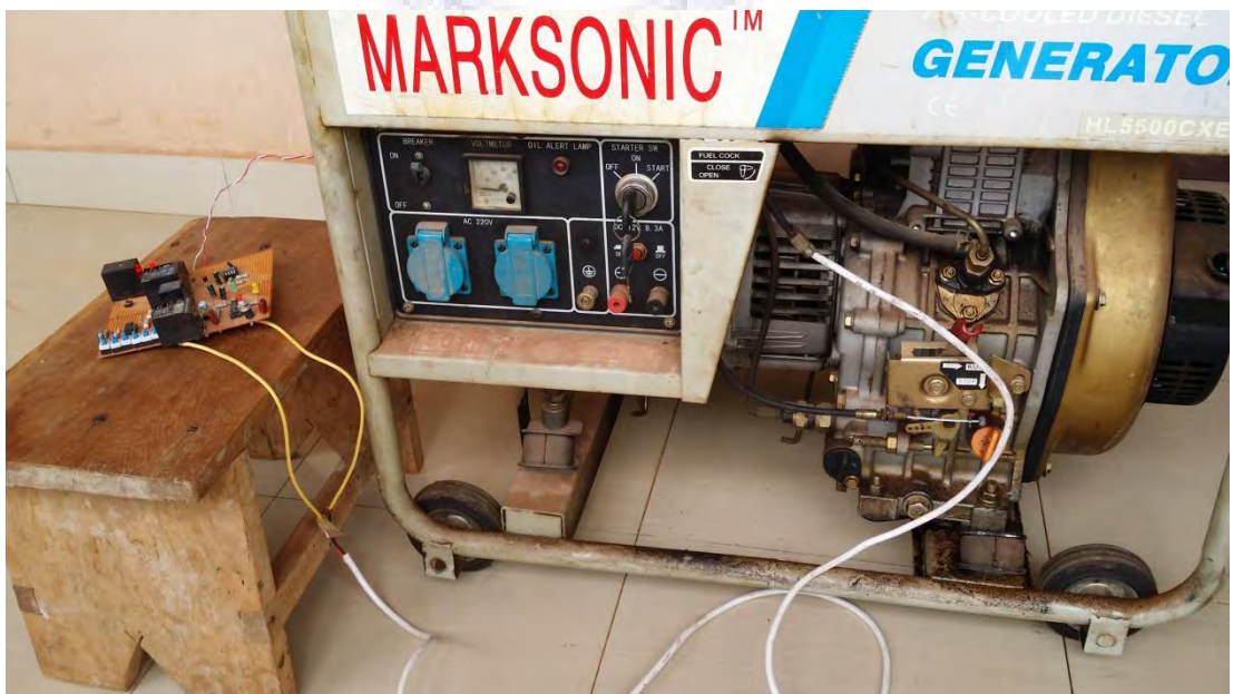
A picture showing the Timer Switch Connected to the Generator Starter or Key to switch of the when the time is due and also and when the fuel finishes.
