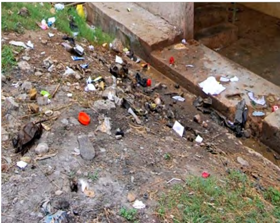
Plate 4.5: Clogged drain system that breeds insects in Salvation A and B Basic Schools
