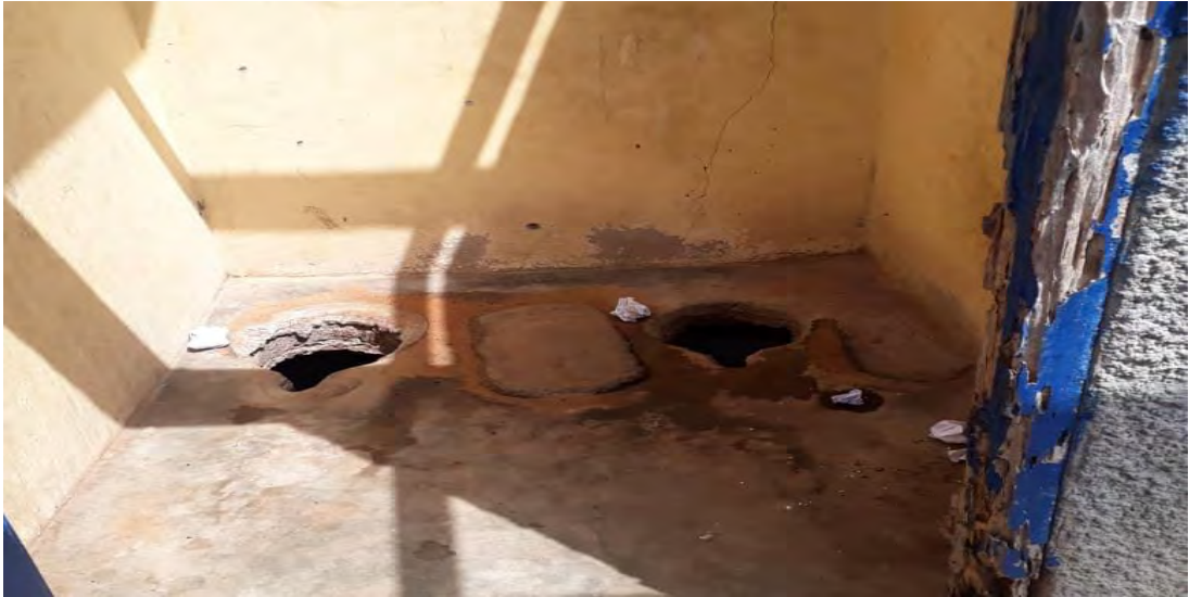
Plate 4.2: A typical toilet facility used in Methodist D/A Basic School
