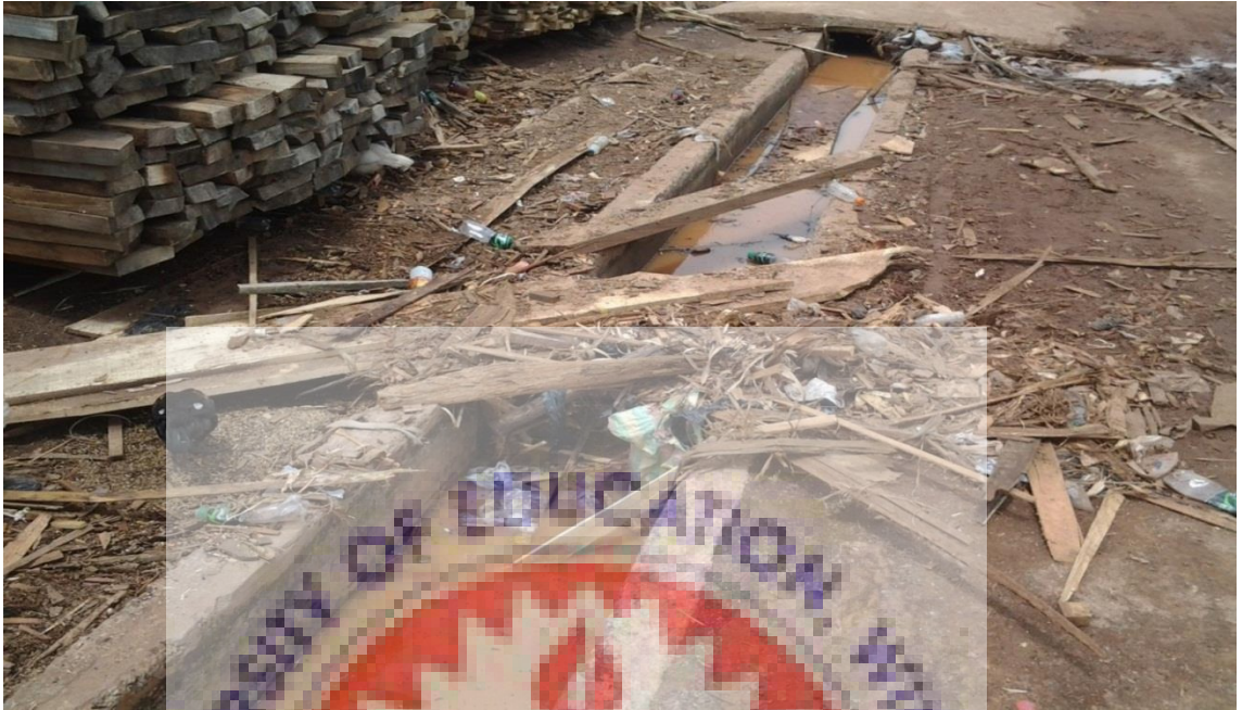
Plate 4.7: Choked gutter by wood waste
