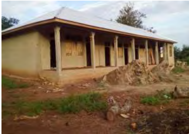
Figure 4.1: Classroom under construction with OPC and Pozzomix cement sandcrete blocks at Aprade construction site.
