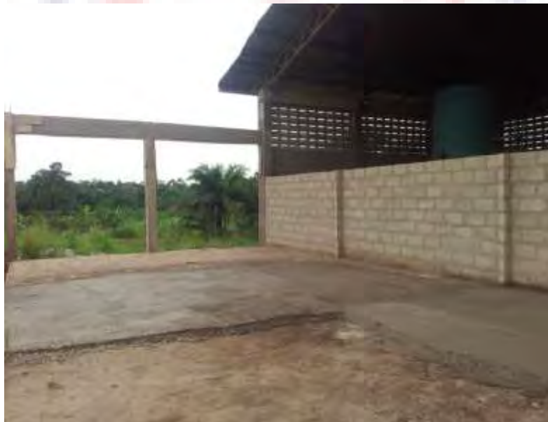
Figure 4. 6 : Picture of pozzomix cement factory under construction with pozzomix cement sandcrete blocks for pozzolana factory at BRRI-CSIR, Fumesua.
