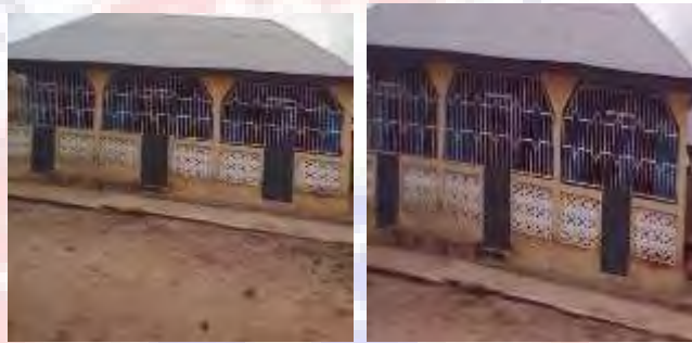
A front view of a structure constructed with OPC sandcrete block at Aprade
